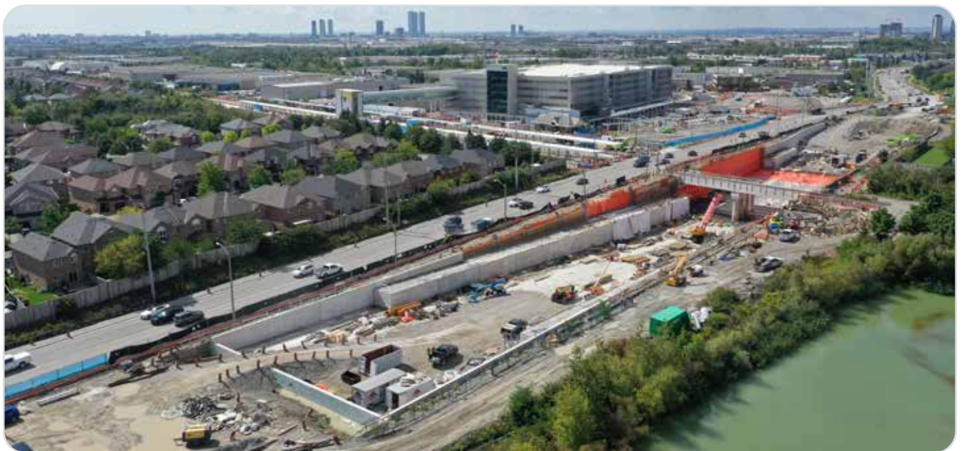
▲ Construction of Rutherford GO rail grade separation on Rutherford Road in the City of Vaughan.
