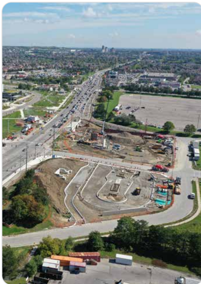
▲ Early phase of construction of Major Mackenzie Drive West bus terminal near Canada's Wonderland in the City of Vaughan.
