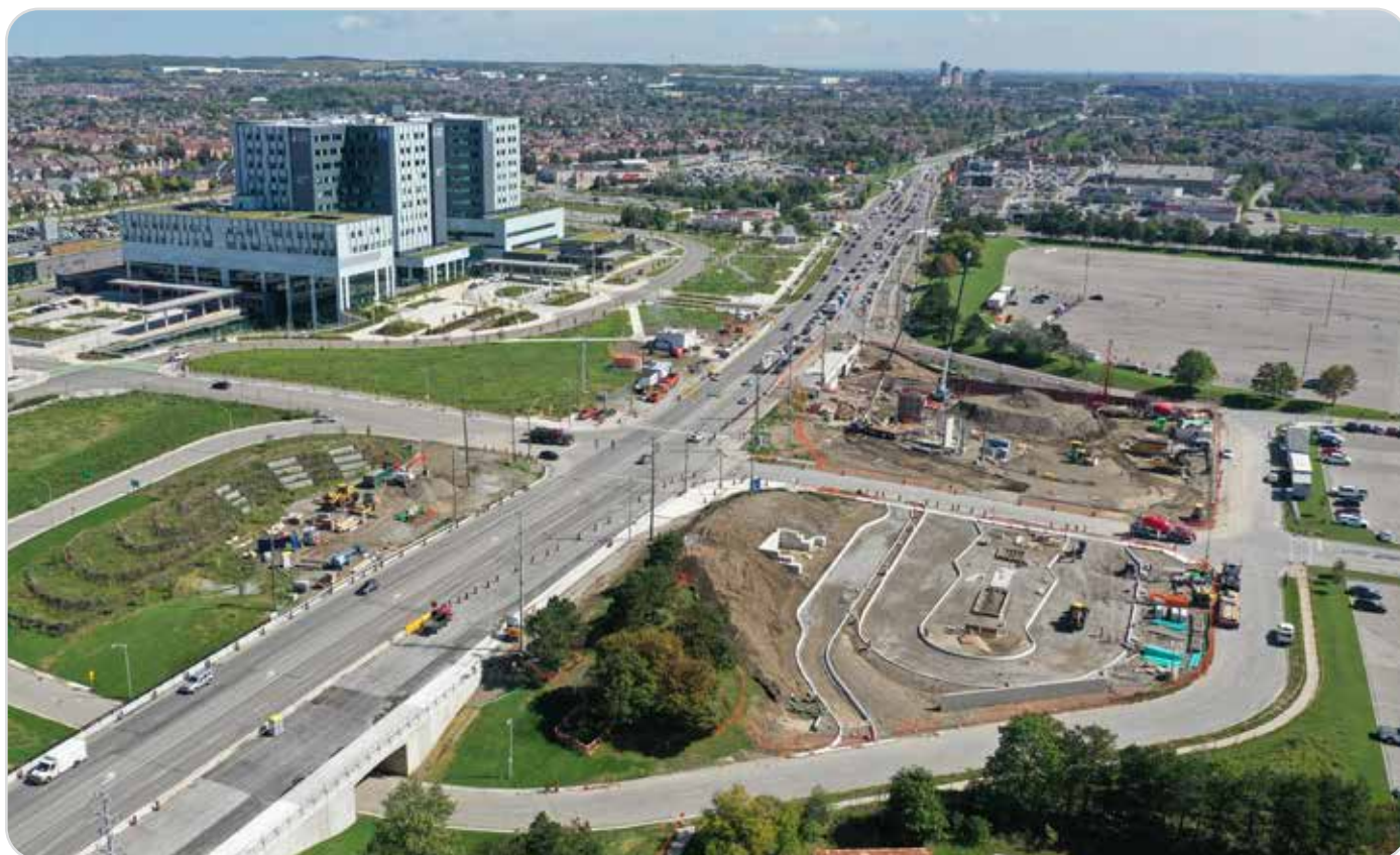
▲ Early phase of construction of Major Mackenzie Drive West bus terminal near Canada's Wonderland in the City of Vaughan.
