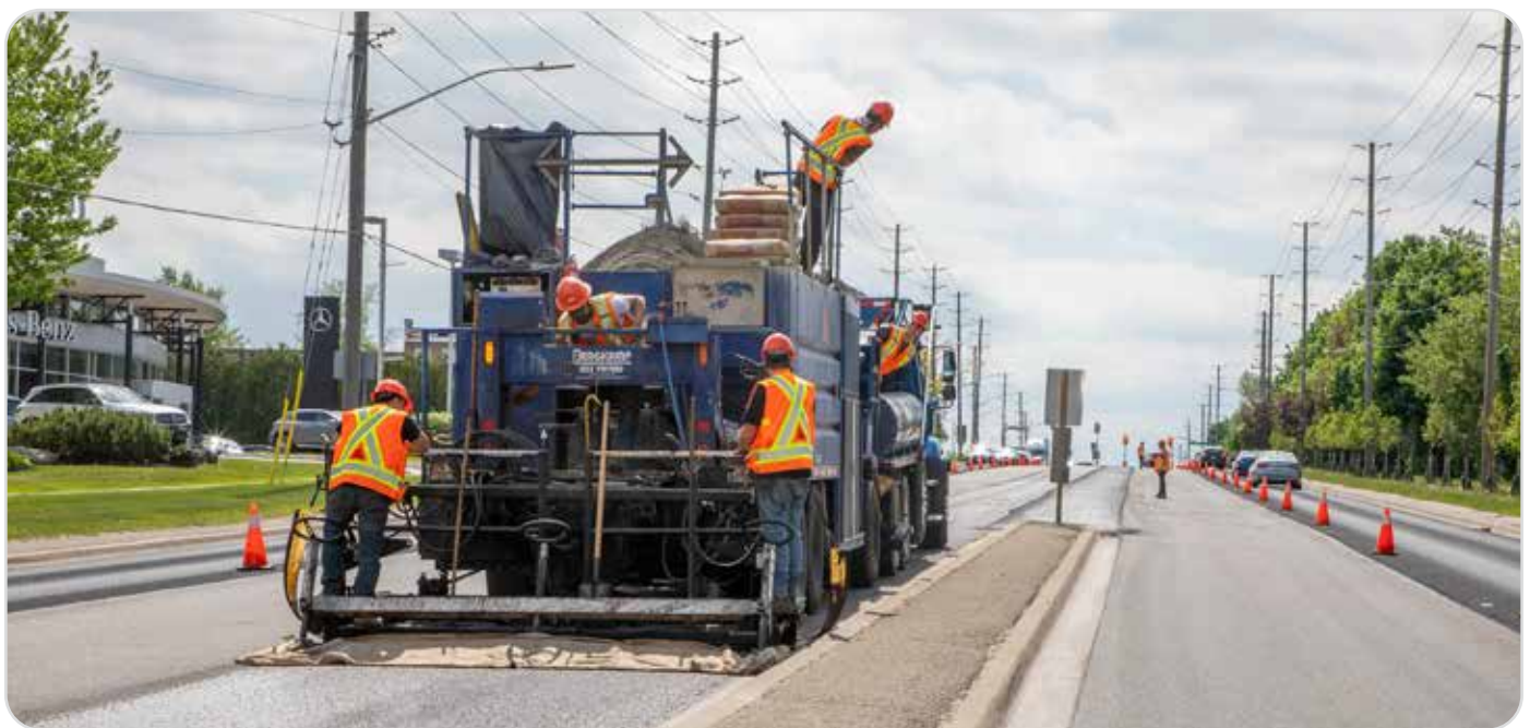
▲ Resurfacing of Mulock Drive, East of Yonge Street in the Town of Newmarket.
