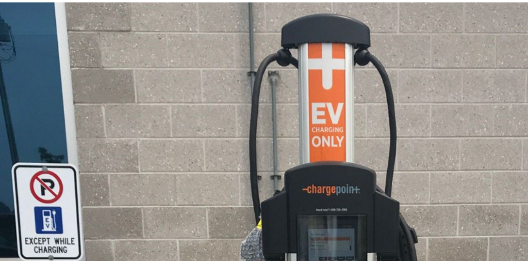
EV CHARGING STATION
