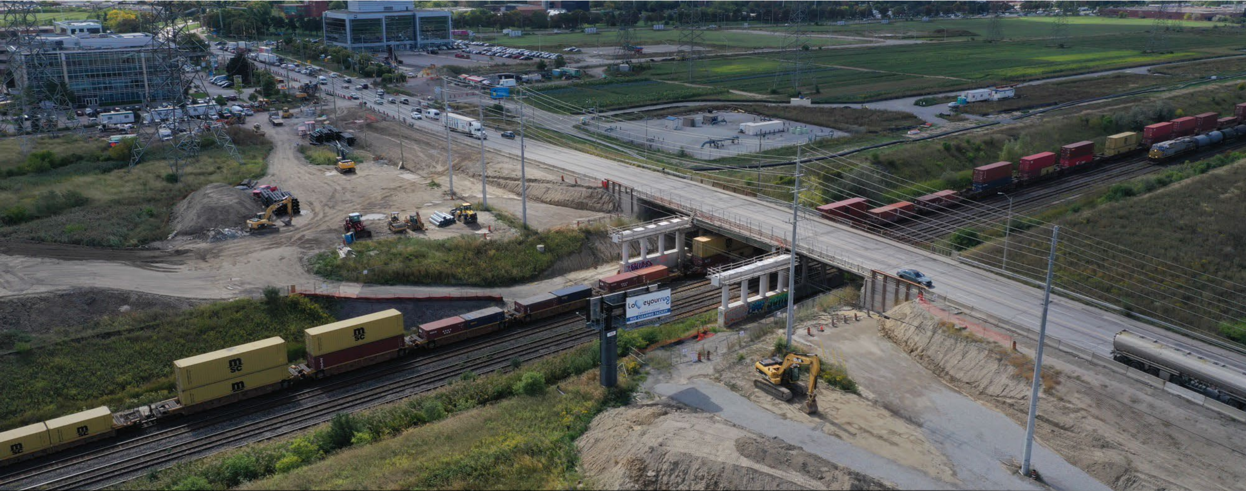
Reconstructing and widening to six lanes, including a new, wider bridge over CN Rail tracks
