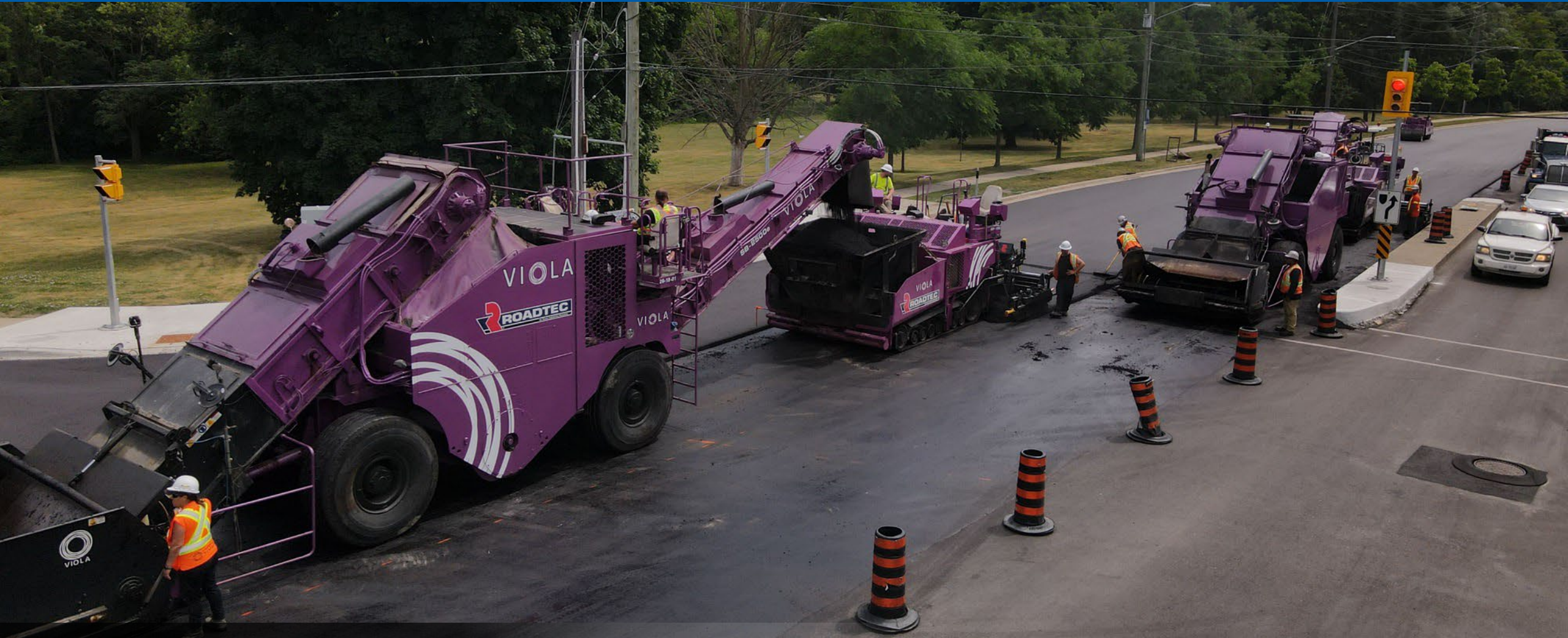
Paving on Islington Avenue between Highway 7 and Langstaff Road, City of Vaughan
