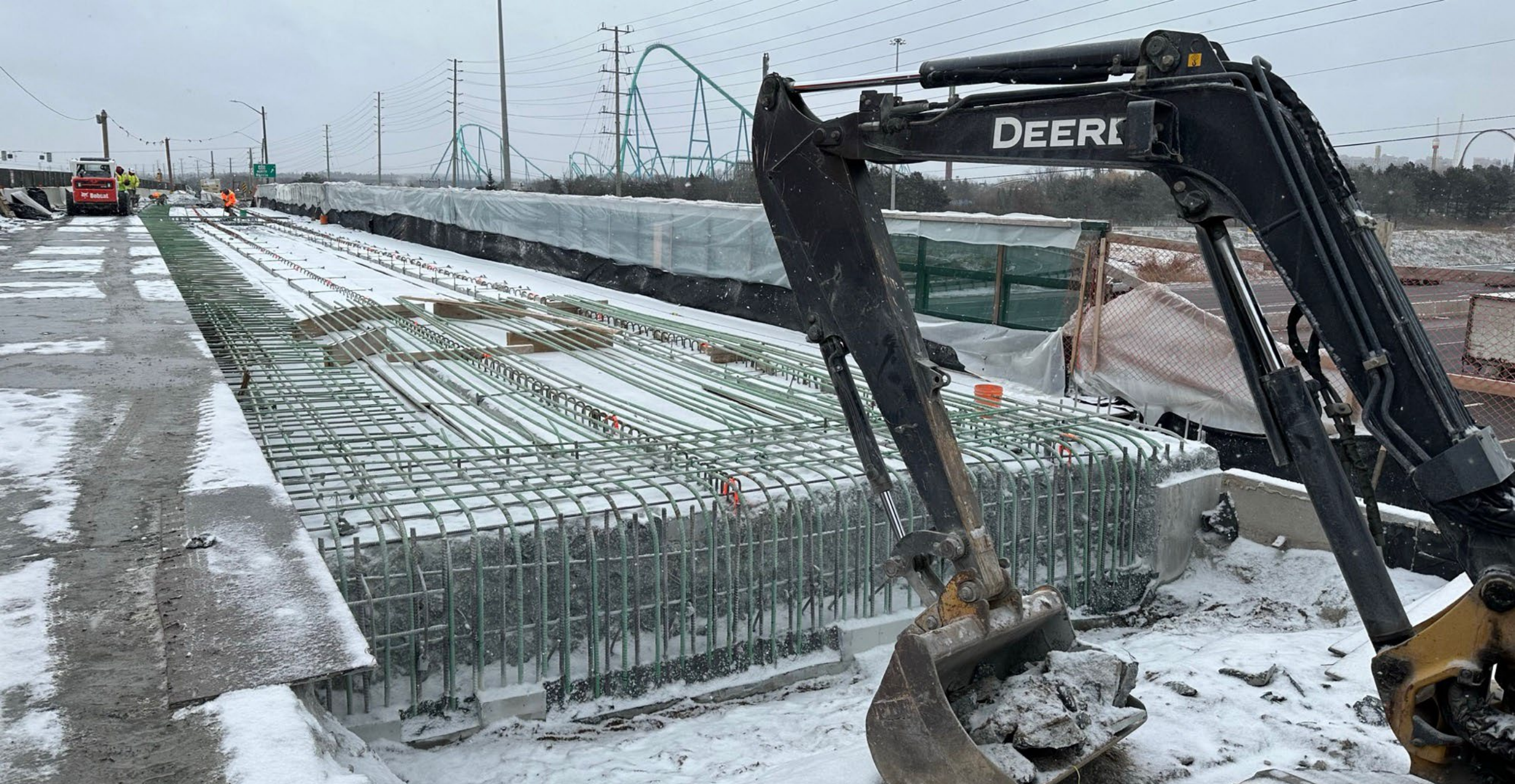
Widening of the bridge on Major Mackenzie Drive over Highway 400 to accommodate a new multi-use path
