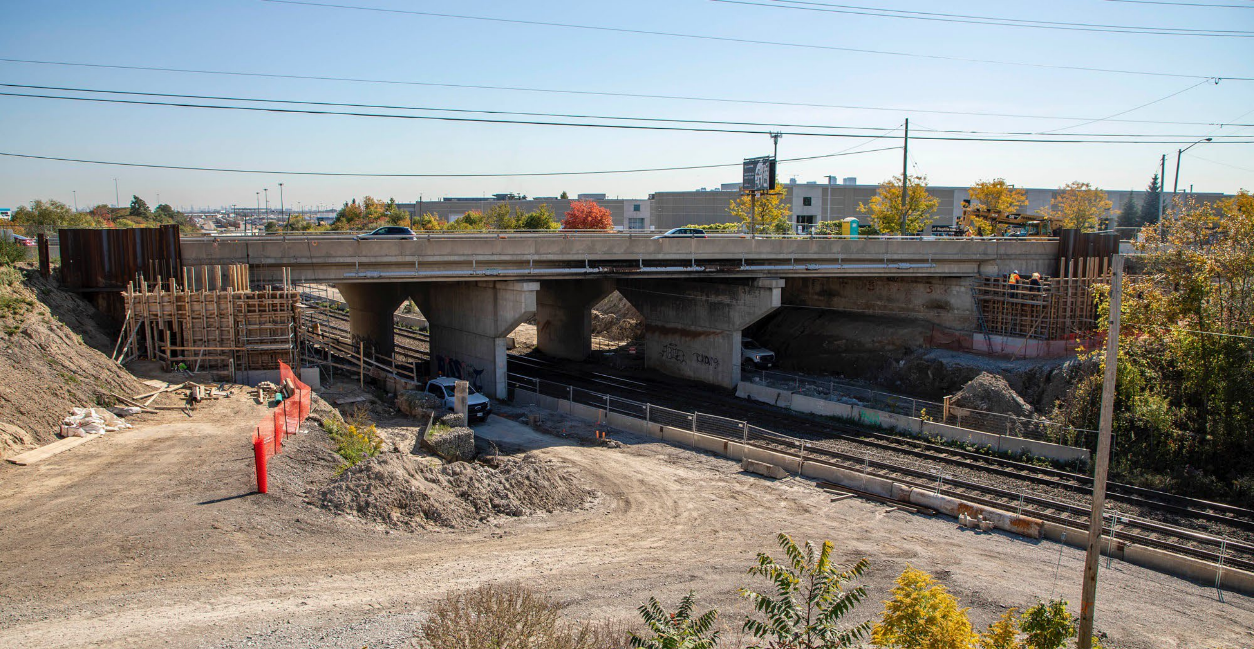
Widening the existing bridge over CN Rail tracks into the CN MacMillan yard
