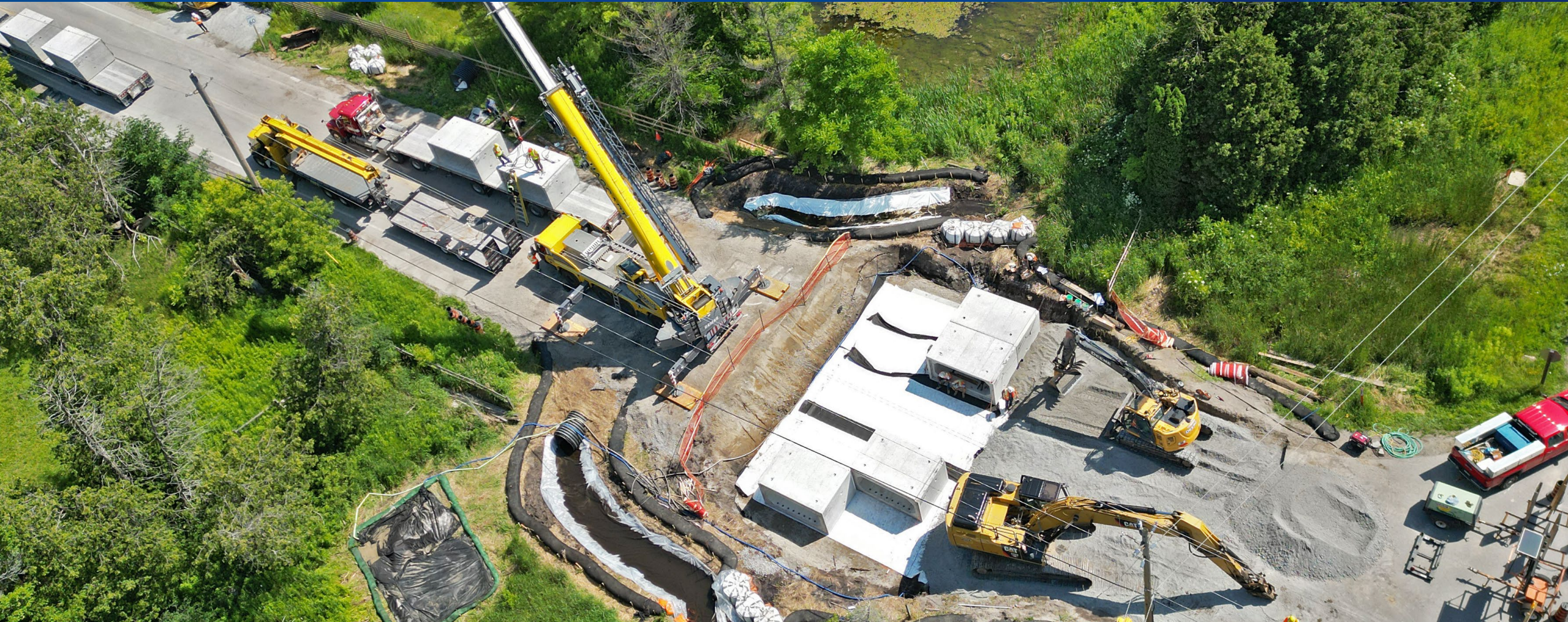
Culvert replacement on Kennedy Road, north of Vandorf Sideroad, Town of Whitchurch-Stouffville
