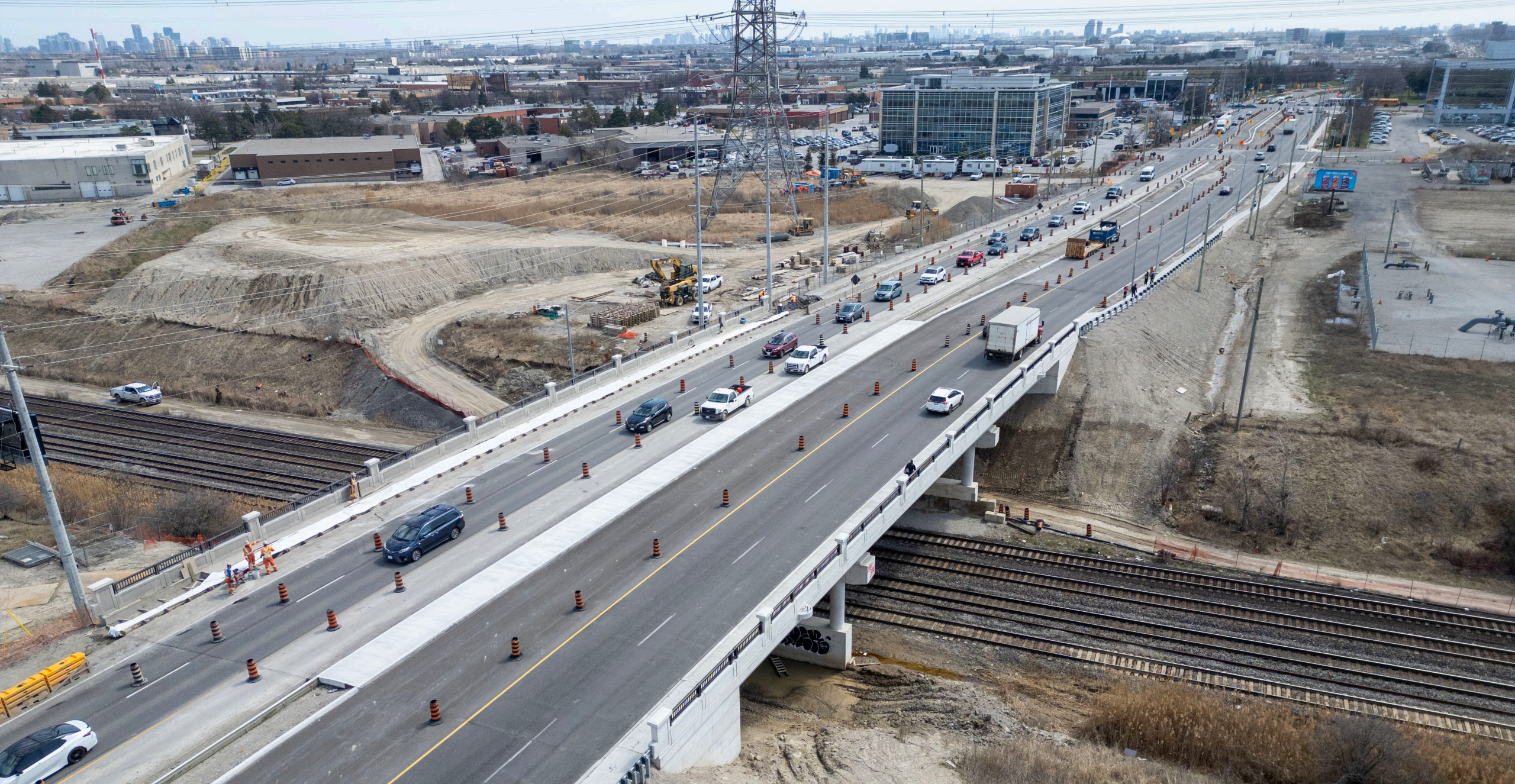
New and widened CN Rail bridge on Keele Street, City of Vaughan
