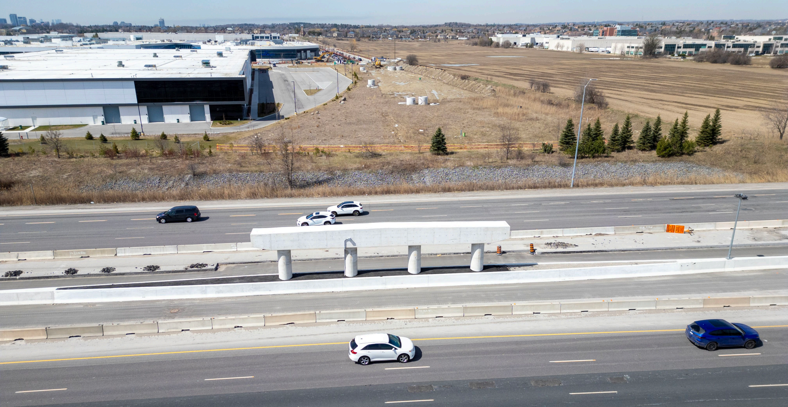
Centre pier for new bridge over Highway 404 constructed by MTO on behalf of the Region, Cities of Markham and Richmond Hill
