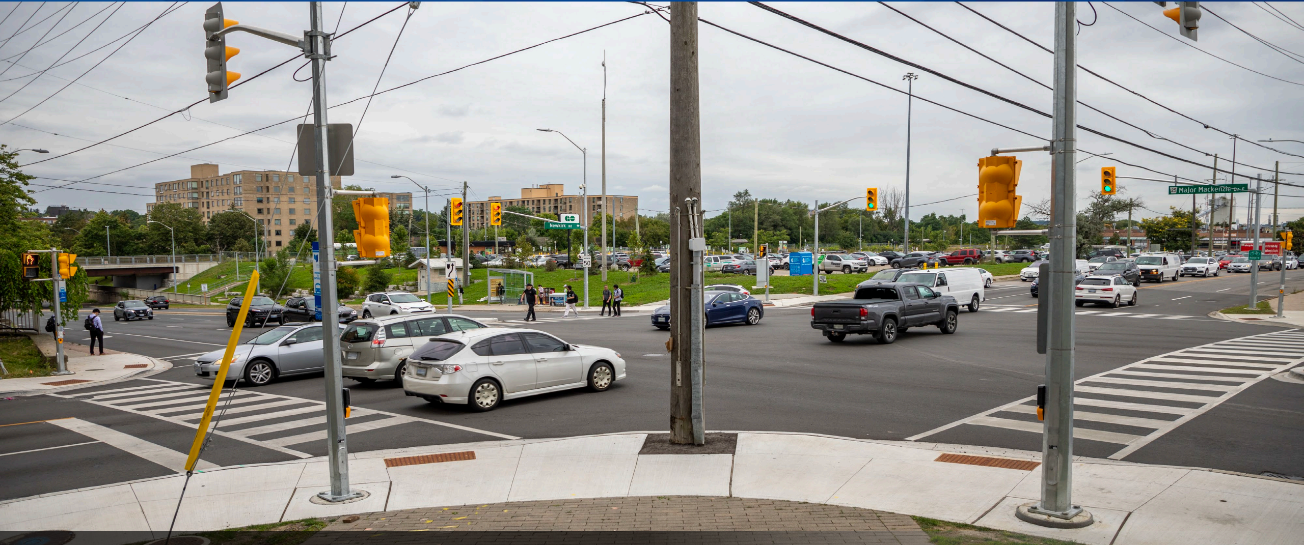
Intersection improvements completed at Major Mackenzie Drive and Newkirk Road / Essex Avenue, City of Richmond Hill
