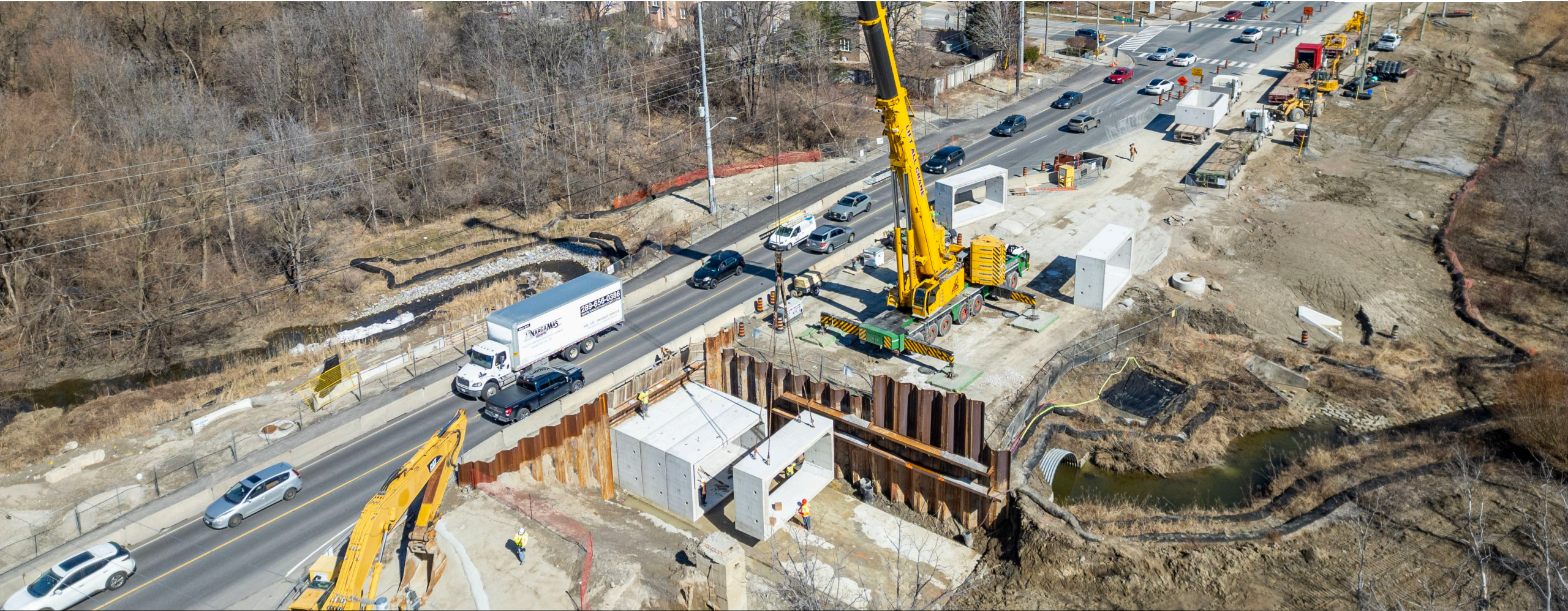
Road rehabilitation, reconstruction and widening from four to six lanes, including a new, wider bridge over CN Rail tracks, City of Vaughan
