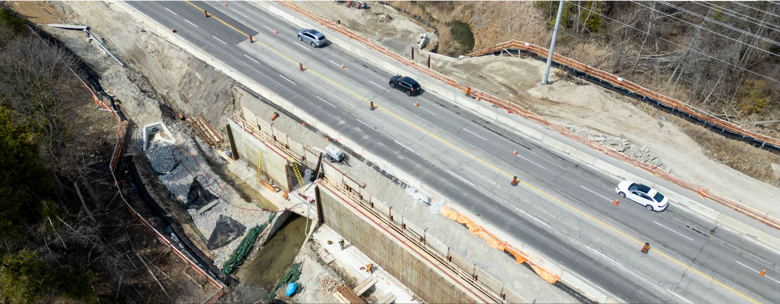
Road widening from four to six lanes, including installing a multi-use path, sidewalk, illumination and streetscaping, City of Vaughan
