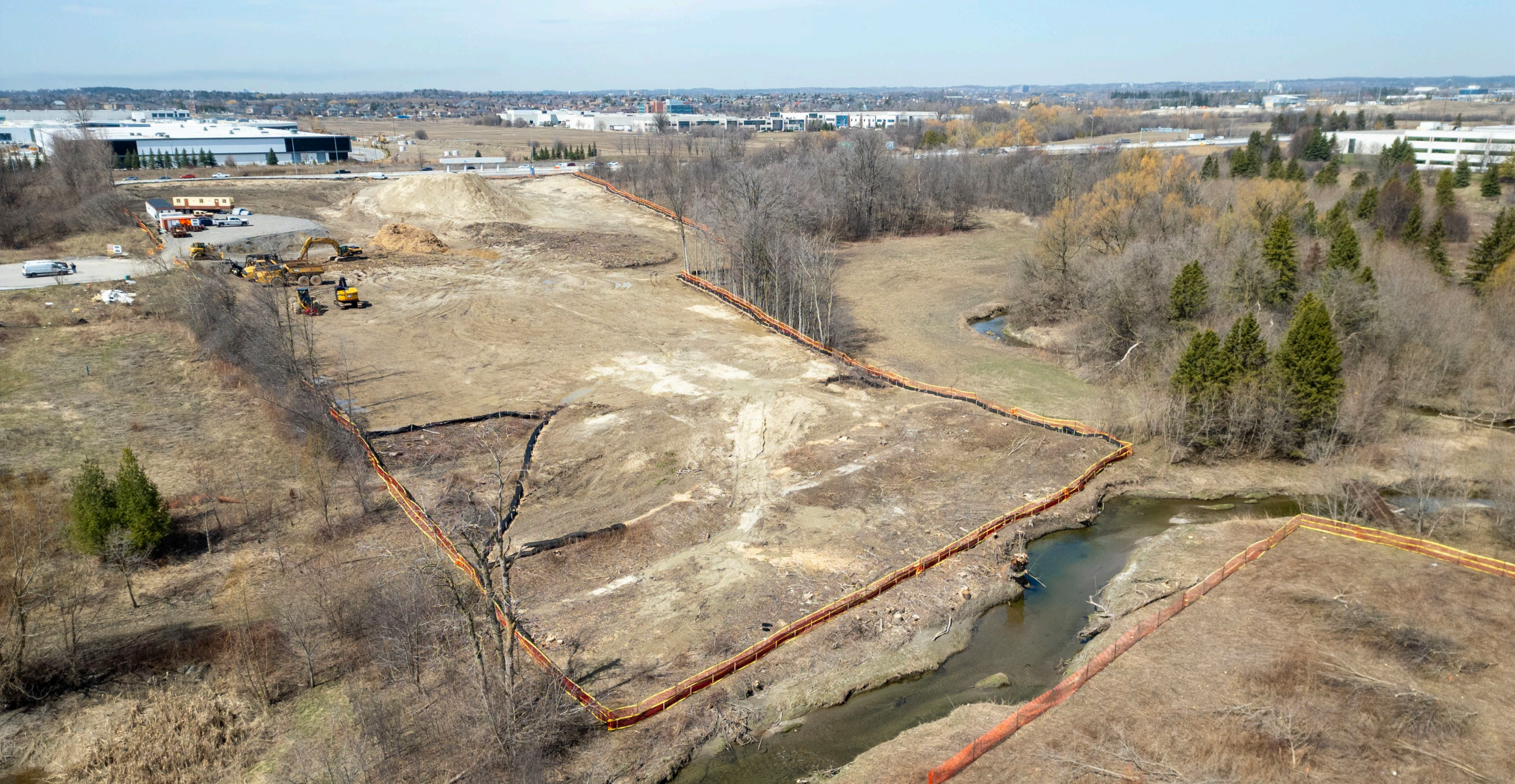
Preparation underway for roadway and bridge construction, looking west toward Orlando Avenue, Cities of Markham and Richmond Hill
