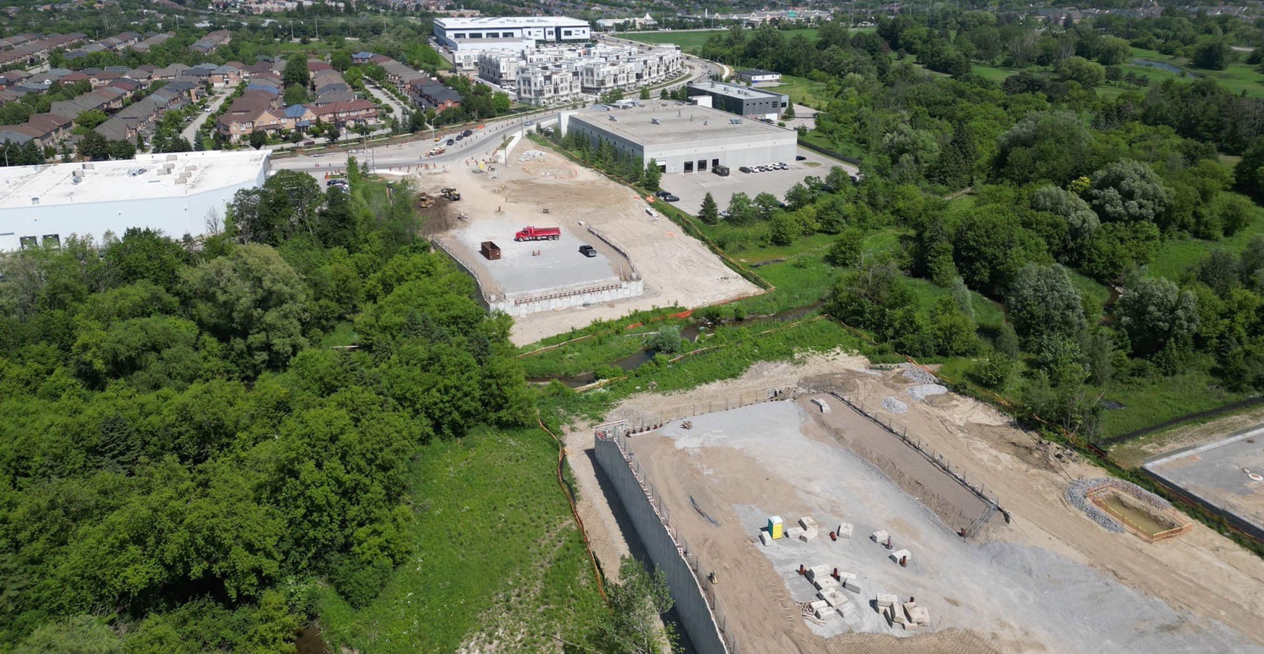
Preparation for girder installation on new bridge over Rouge River, west of Markland Street, City of Markham
