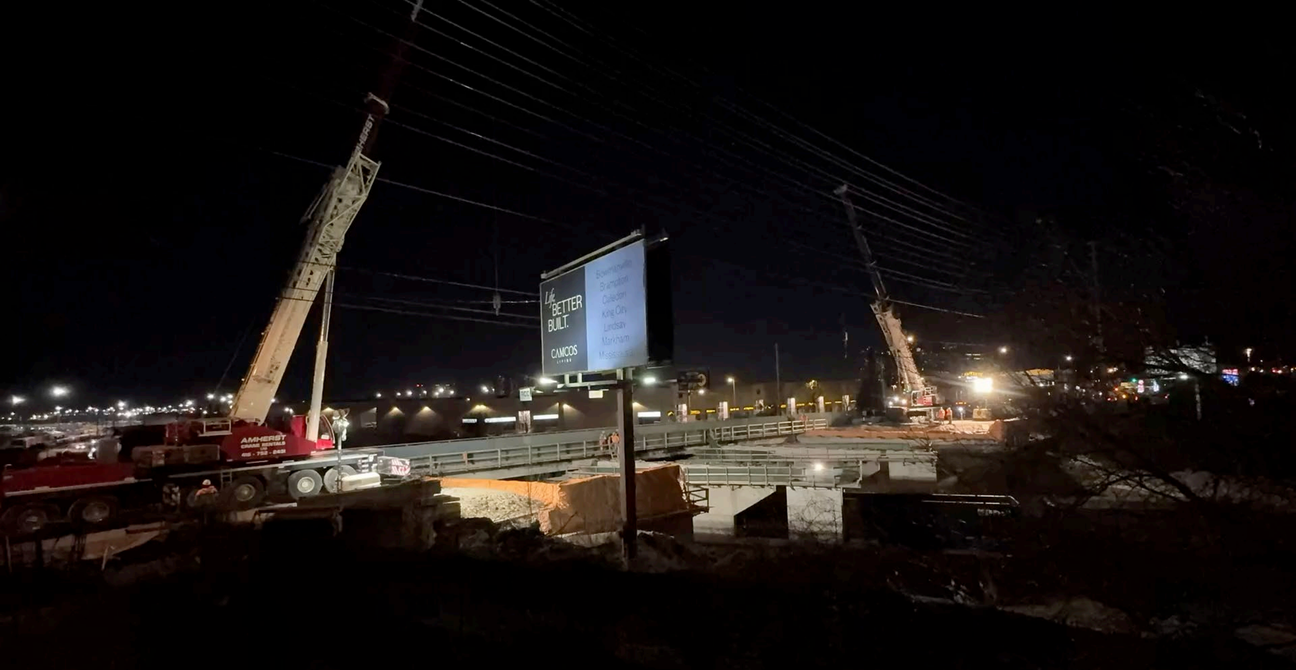
Timelapse of girder installation for CN Rail bridge on Rutherford Road, east of Melville Avenue/Creditstone Road, City of Vaughan
