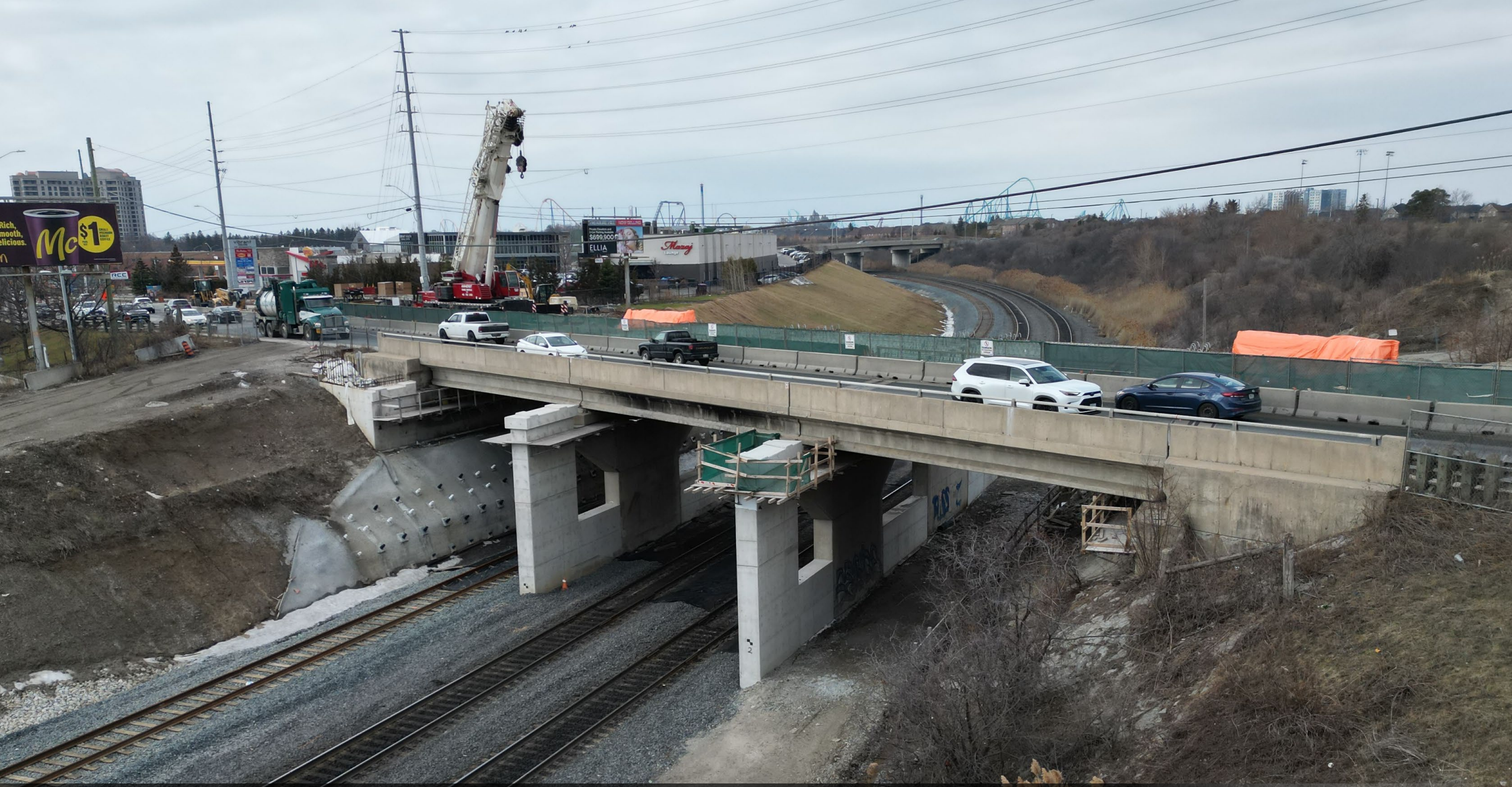
Track level work complete for CN Rail bridge on Rutherford Road, east of Melville Avenue/Creditstone Road, City of Vaughan
