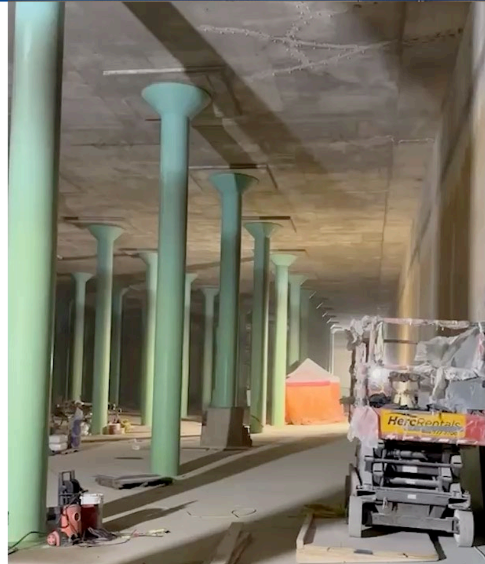
Inside the South Maple Reservoir, City of Vaughan
