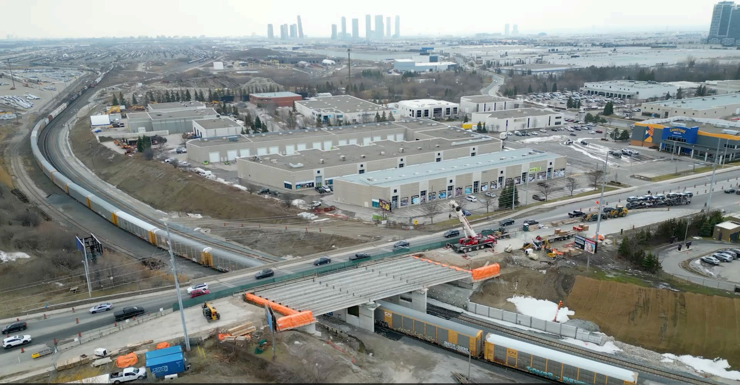
Aerial view of the CN Rail bridge on Rutherford Road, east of Melville Avenue/Creditstone Road, City of Vaughan
