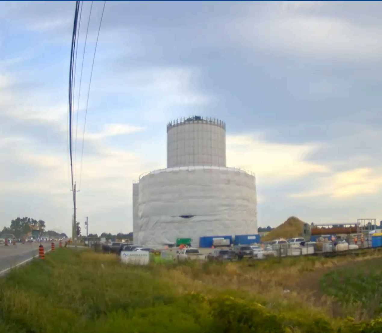
Northeast Vaughan Water Servicing, Elevated Tank and Pumping Station, City of Vaughan
