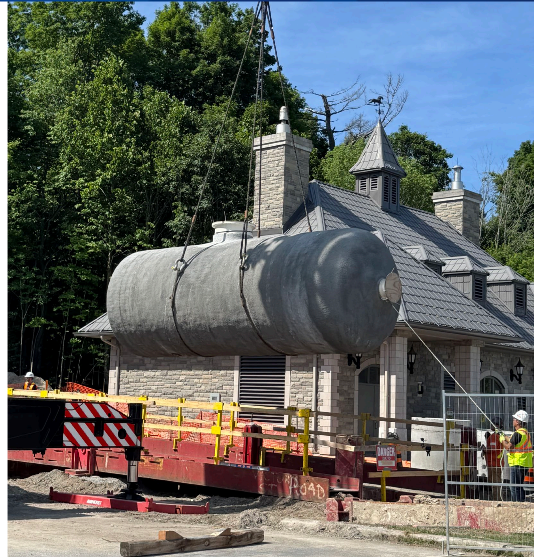
Chlorine tank installation at Ballantrae Wells 3 and 4, Town of Whitchurch-Stouffville
