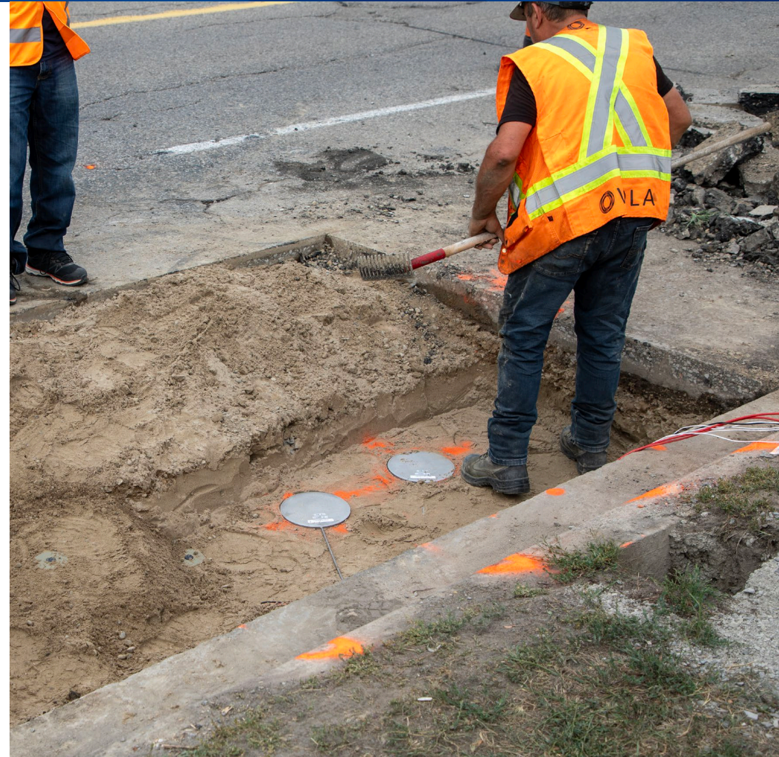
Installation of sensors for high RAP trial Leslie Street, City of Richmond Hill
