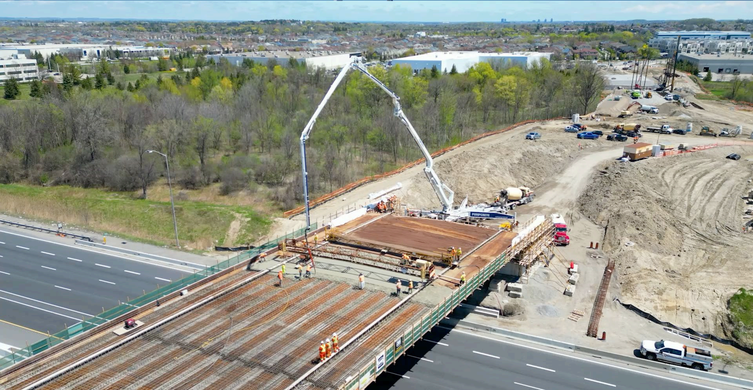
Concrete pouring underway on bridge over Highway 404, looking east toward Markland Street, City of Markham
