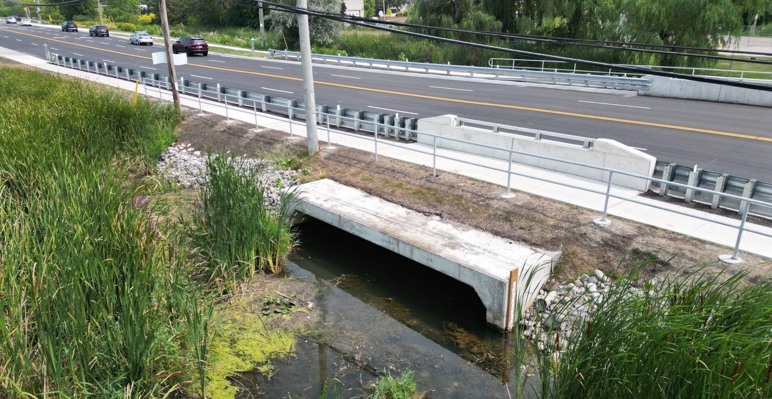
New culvert on King Road, west of Yonge Street, City of Richmond Hill
